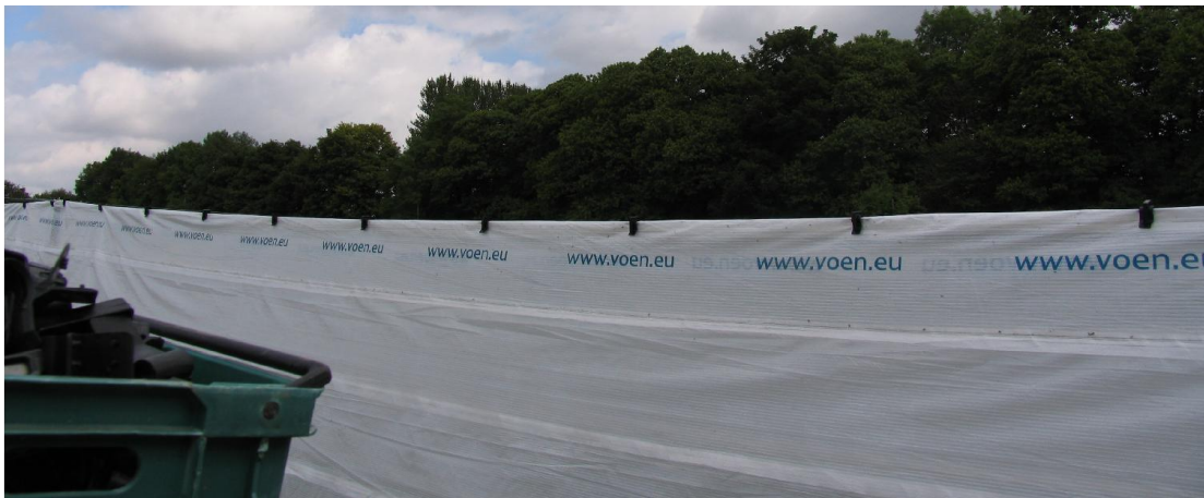
Picture 3: 12 to 13 clips are used between two poles. Use „u“ to „u“ from “www.voen.de” as a guide for the distance of 0,8 metre.
